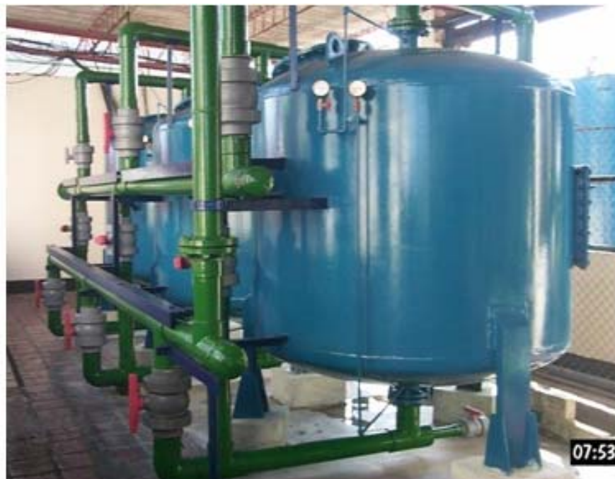
Figure 6. Overview of a filtration system.
