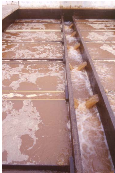
Figure 14. Washing operation of an open filter.
